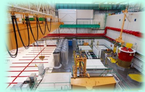
Interim Spent Fuel Storage (wet)
